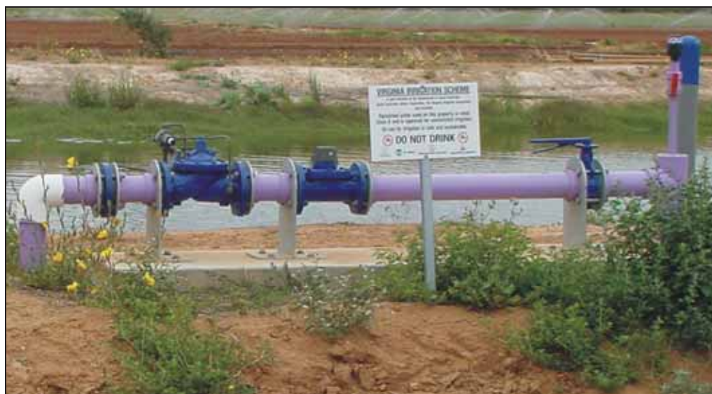
Pipes carrying recycled water are obvious from their lilac colour
